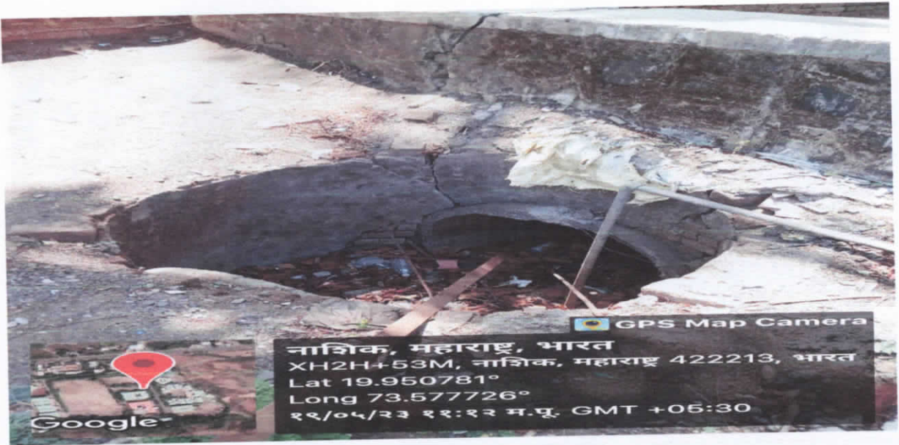
Photograph of Water Drainage system
